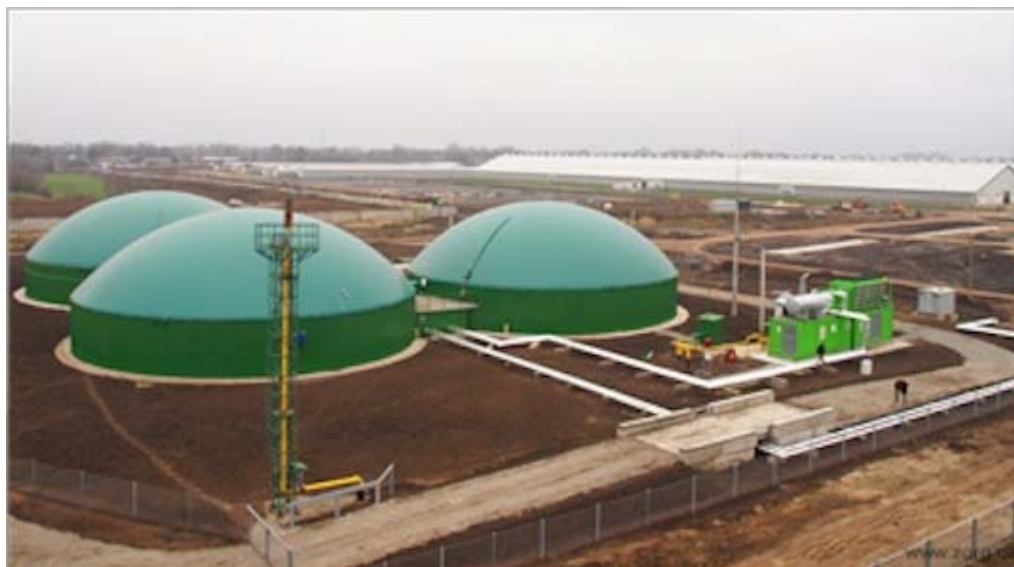
Figure 8: Enclosed Bio Gas Tanks
